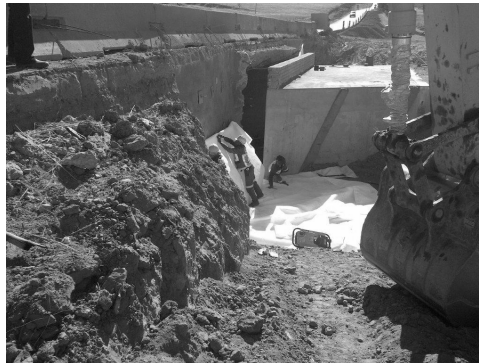
Figure 6. Illustration of shot-creting, new jersey barriers for existing road, new culvert and first layer of geo-synthetic fabric being placed. Captured by Author
