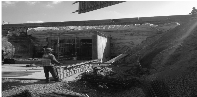
Figure 8. Left hand side new culvert under construction with right hand side at final road level. Captured by Author
