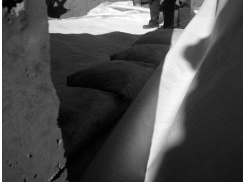
Figure 6. Sand bags placed along edges of vertical face to provide additional stability during the compaction process. Captured by Author
