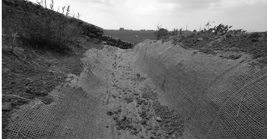
Figure 7. Erosion control blank on slope drain.
