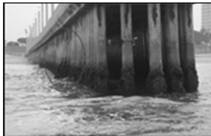
Figure 6: Failure of the piles (CSCM)
