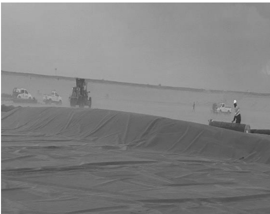
Figure 2. Wind beneath the liner caused by insufficient anchoring.
