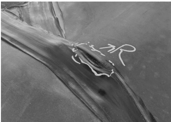
Figure 6. Burn out due to improper temperature control and inconsistent welding speed (extrusion welding)
