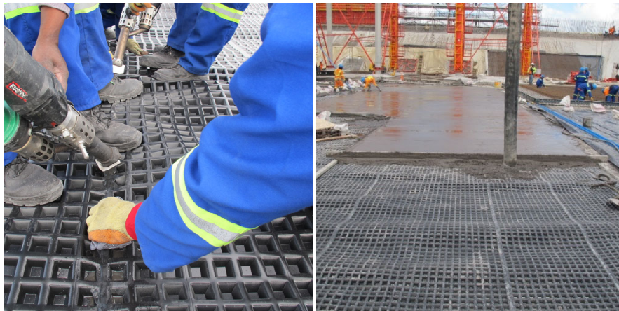
Figure 8: a) Extrusion welding of cuspated sheet; b) screed placement onto cuspated sheet.
