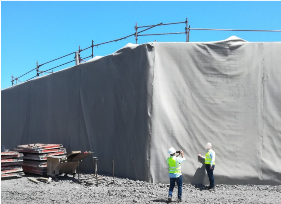
Figure 9: Heavyweight protection geotextile installed onto 2mm HDPE liner along the sides of the retaining walls of the tanks.
