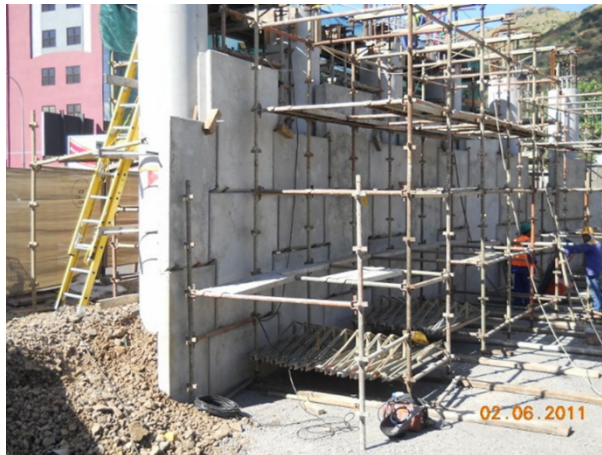
Figure 1. MSEW with bridge piers – issues during construction
