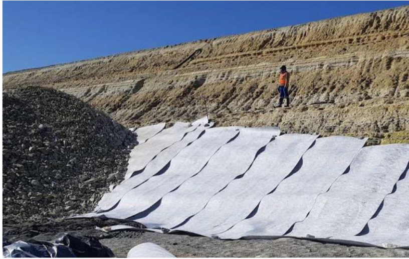
Figure 6: Geocomposite drainage blanket laid on the TSF slopes in the non-critical areas.
