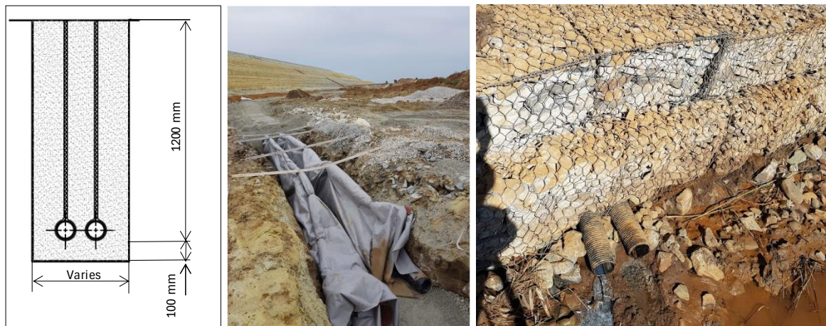
Figure 2: HDPE drainpipes, (left) typical drawing section, (middle) site installation, and (right) post-construction monitoring.
