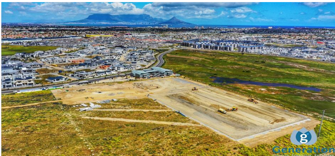
Figure 8. Sports Complex Earthworks Under Construction. The Project Looks Over the Sandown Fynbos Corridor and the Sunningdale Ephemeral Pan.
