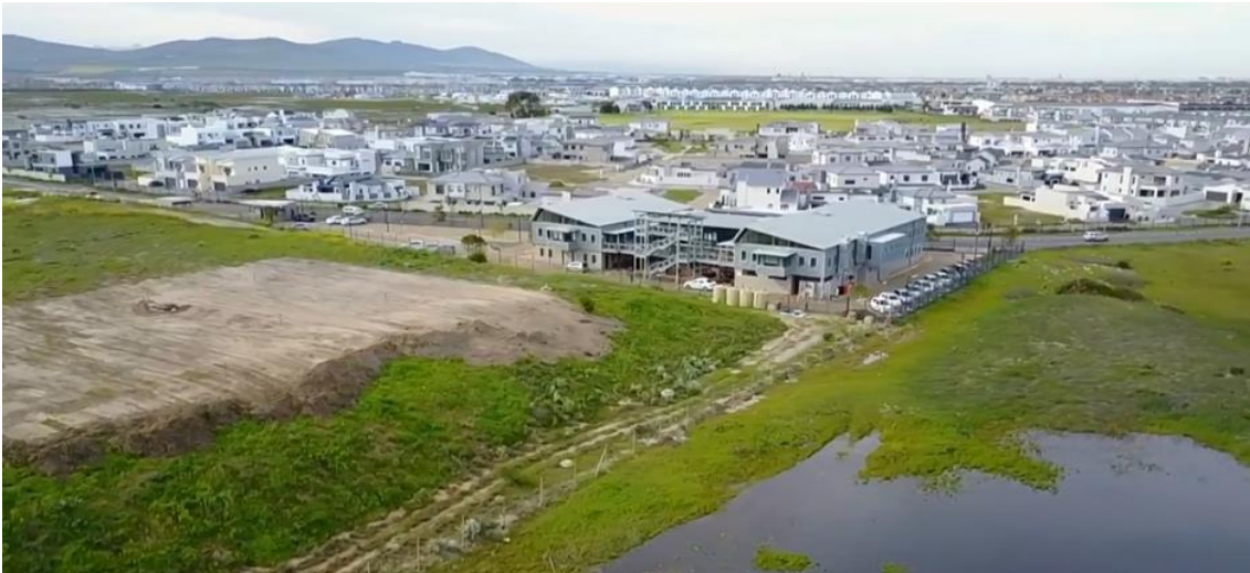
Figure 7. Clearing Work on the Landfill Begins, Sunningdale Ephemeral Pan Wetland in Right Bottom Foreground
