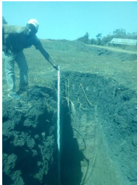
Figure 2. Depth of black cotton soil at road section (Image source: Nabaki Afrika, 2017).
